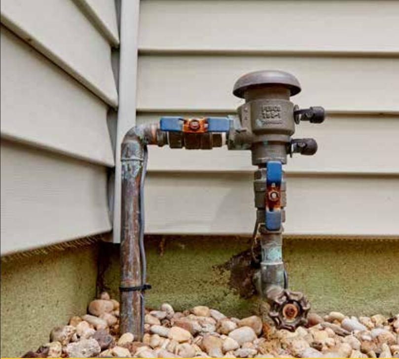
SPRINKLER SYSTEM BACKFLOW ASSEMBLY
